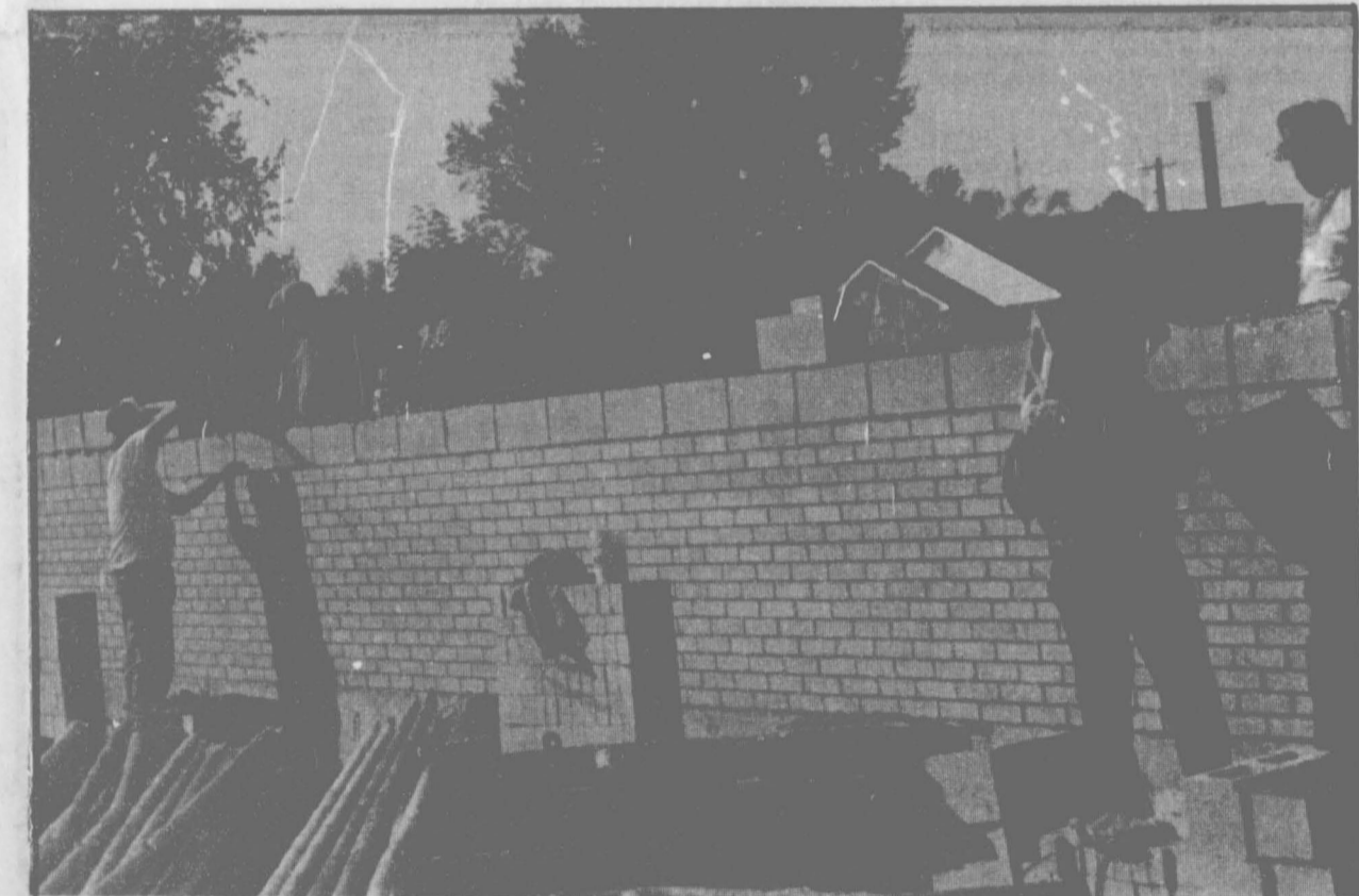
If you haven't driven by the Elementary School Building lately, you should. There has been a lot of progress made lately. The most noticeable is that of the brick laying. The bricks are going up quickly.
