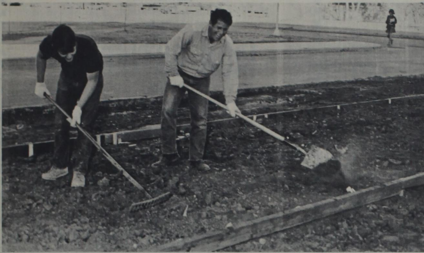
NEW SIDEWALKS —Grounds maintenance workers Bruce Zoller and Richard Anderson prepare ground around the BA Building for new sidewalks which are
