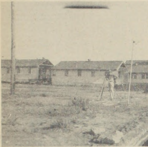
TAKE IT AWAY—Construction workers are shown above as they begin making preparations to remove one of the army surplus or X buildings on the Tech campus which have served as classrooms for the past two years. The buildings are being torn down to make room for permanent installations now being built. (Photo by Lee.)
