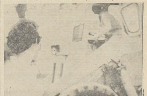
COMING THROUGH—a Tech student watches the new construction work being done to add parking lots for the girls' dorms.
