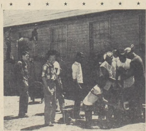
SEEING GREEN?—Los Camaradas members and pledges paint the Rec hall its original green color as no red paint was available. A day's work was spent by the Cams, painting and scraping the building. (Dolores Ketchersid Photo)
