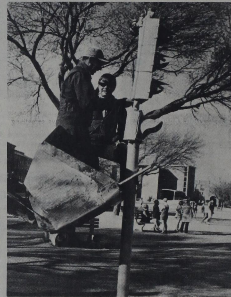
REMOVAL BEGINS —Workers disassemble traffic lights around Memorial Circle which are no longer needed since the street around the circle has become one-way. (Staff photo by Bruce Ott)
