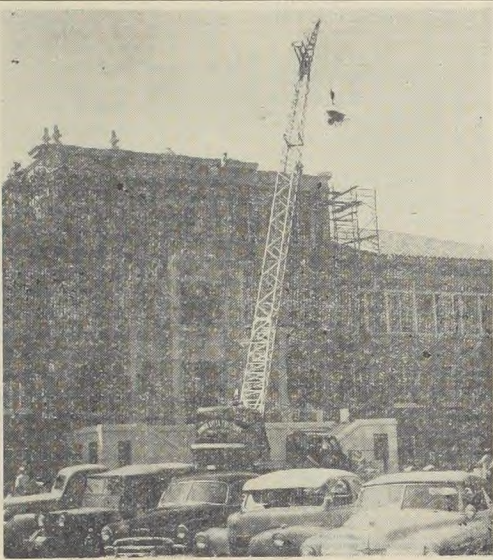
CARTHAGE COMES TO TECH—Three days' work with this crane will be required to do the job of setting stone decorations in place on the front of the new Science building. The sections of cast stone make up a Carthaginian-type design, reports Contractor Allie Hughes.
