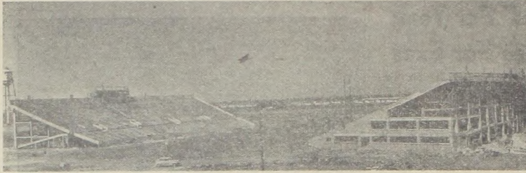
WHEN THE UNBELIEVABLE HAPPENED—Oil-soaked concrete comprising reinforcing forms for Tech's new Jones stadium burst into flame at 5 a.m. June 27, 1947 when the structure was half-finished. The blaze destroyed east side stands and delayed completion of the job for some 60 days.
