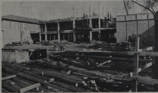
Food and nutrition center A new $4 million structure will be shared by the Colleges of Home Economics and Agricultural Sciences. The Center of Teaching and Research in Food Science and
