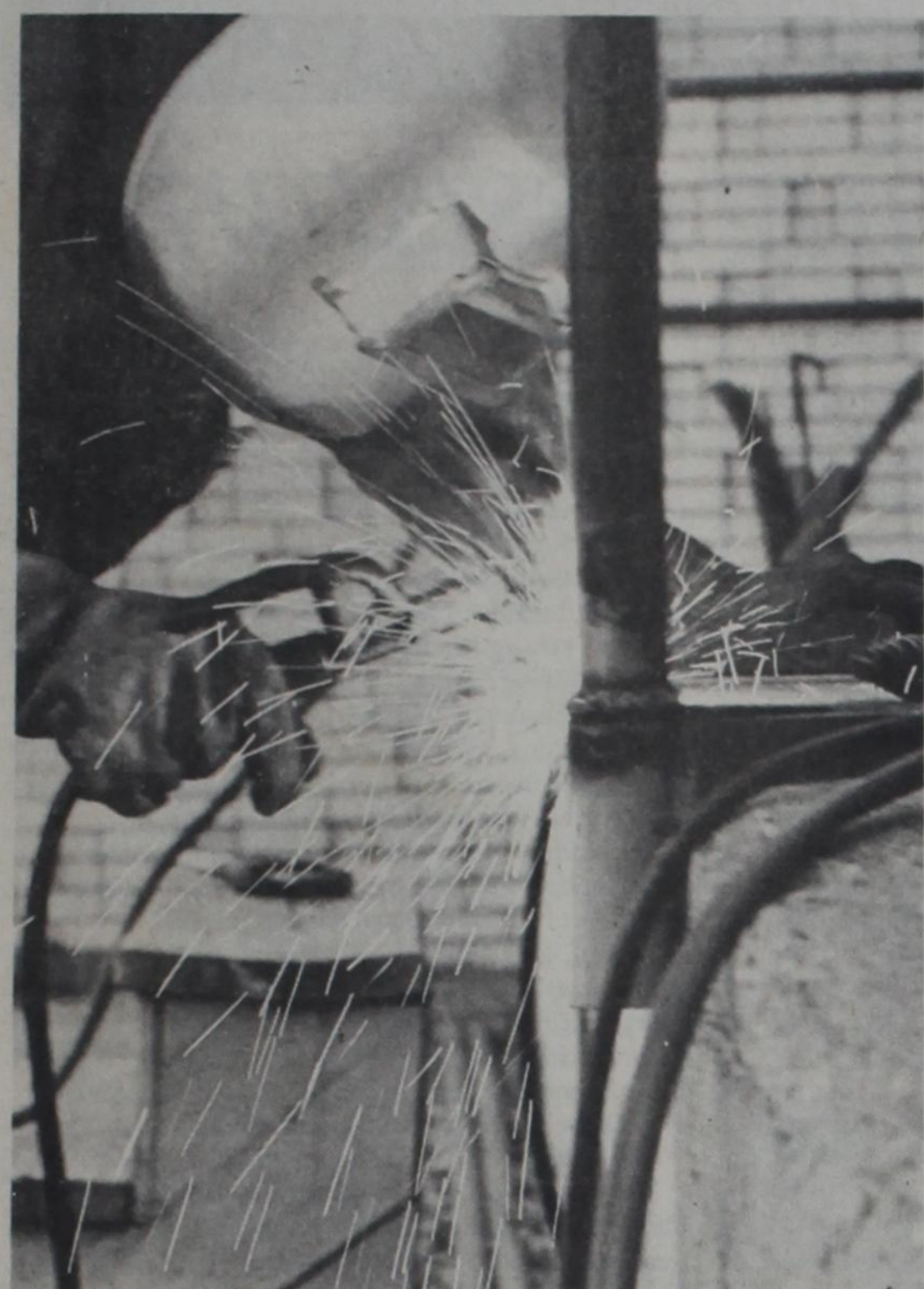
Sparks fly as fire melts metal. James Shaw, a Tech building maintenance worker welds a rail to a ramp outside the Journalism Building. (Photo by Mark Rogers)
