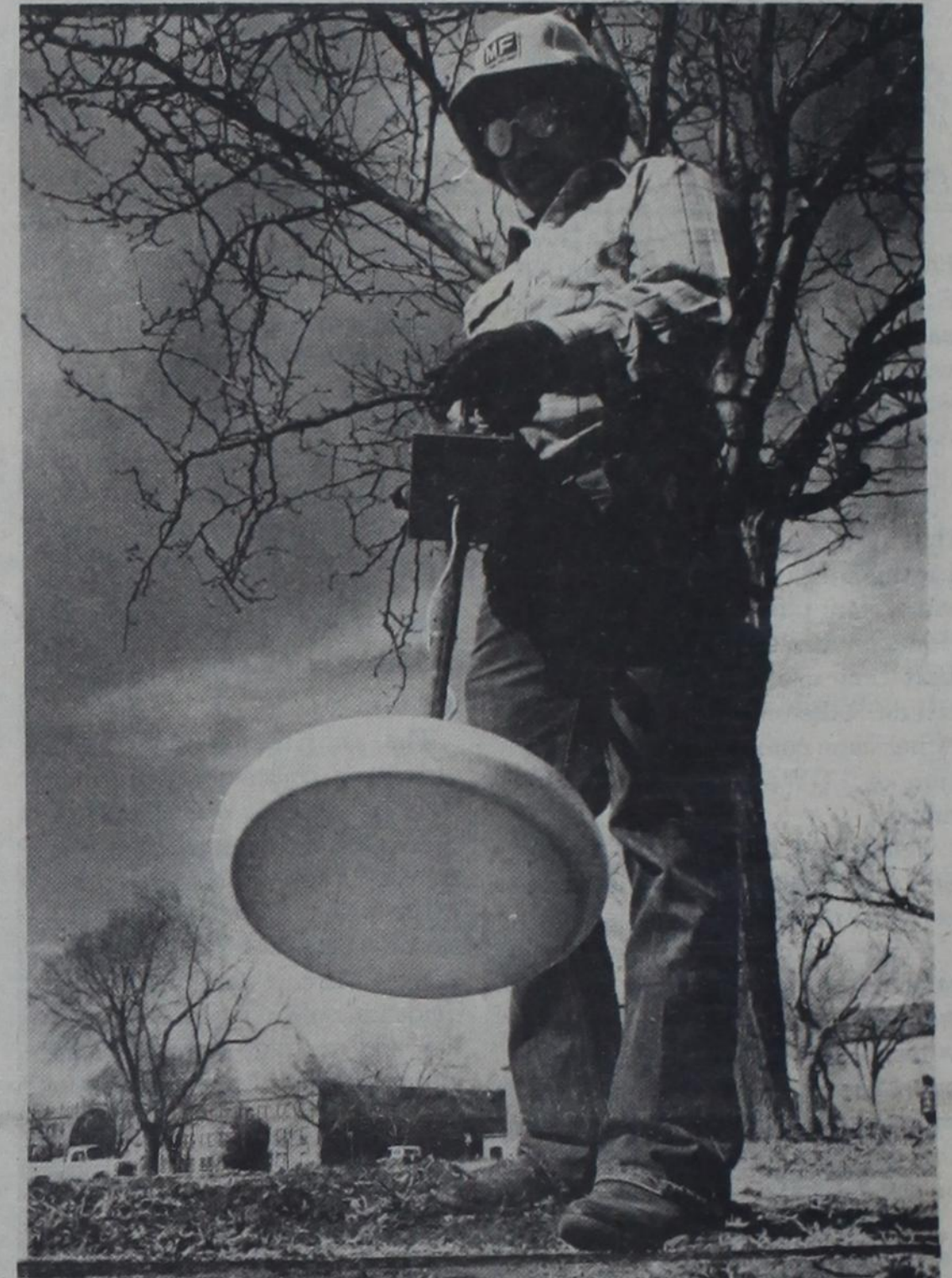
Armando Urrutia of Tech maintenance searches for a water main with a metal detector. The water main is located near Broadway and University Avenue where the excavation is taking place. Behind Armando is a clear, sunny sky that is soon to change today and be replaced by clouds and colder weather. (Photo by Mark Rogers)
