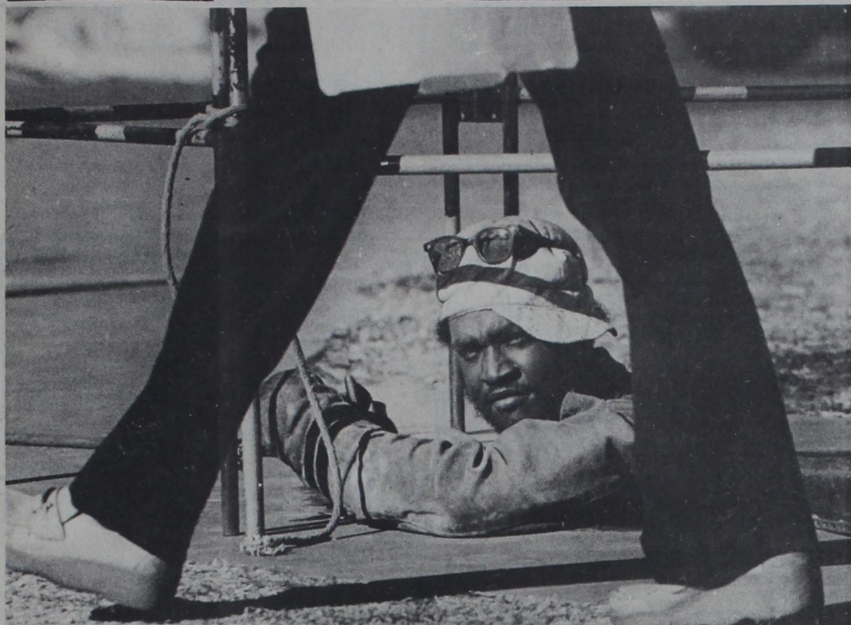
Above, James Shaw of Tech Maintenance breaks from his work to get a breath of fresh air after welding underground. (Photo by Mark Rogers)
