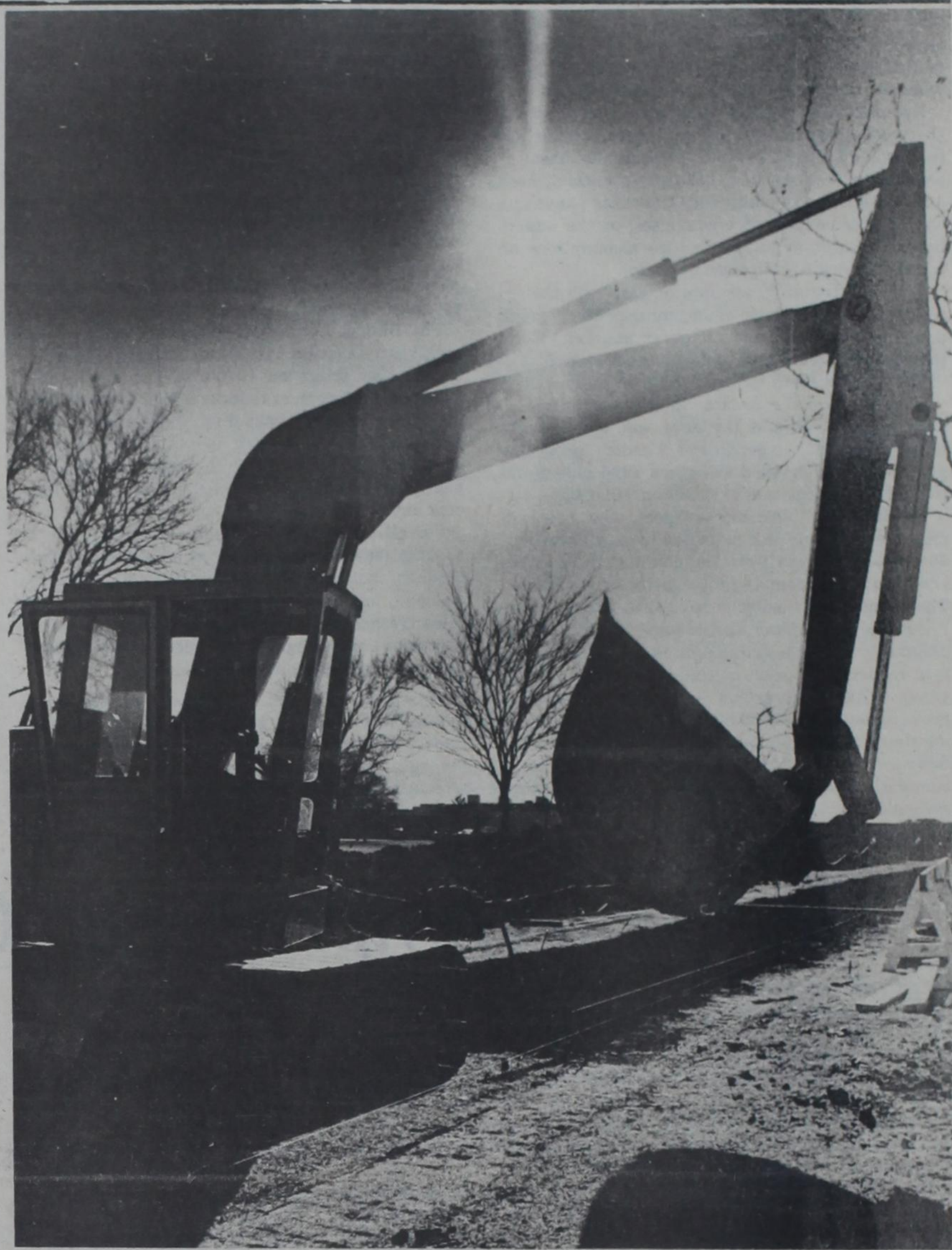
Installation of a heating pipe continues on 6th street. Drivers are advised to seek a detour because excavation is expected to continue today and possibly disturb traffic. Above, the operator prepares to bite another chunk of dirt off of the edge of the evidently deep hole. (Photo by Max Faulkner)
