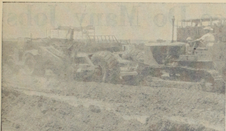
WORK PROGRESSING —Earth moving machinery is pictured preparing ground around the new women's dorm south of the library for paving and landscaping. Work on the structure and grounds is in high in order to have all in readiness for its occupants this fall. —Staff Photo
