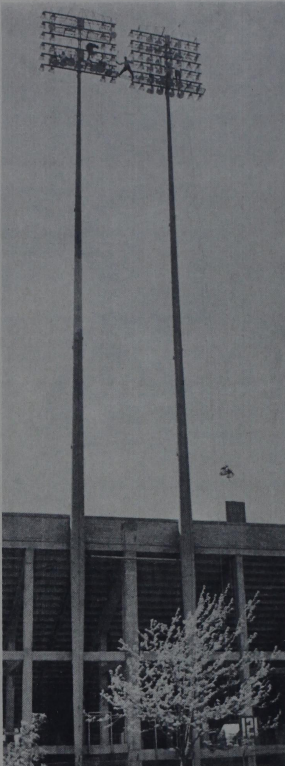
BALANCING ACT? —Workers remove lights in Jones Stadium in preparation for new lights to be installed for the Coaches All-America Game on June 27. (Staff photo by Bruce Ott)
