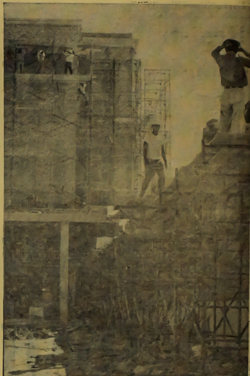
NEW ADDITION TO SKYLINE—The new six-story women's dormitory is a month ahead of schedule. Begun late in May, the structure is slated for occupancy by next summer.
