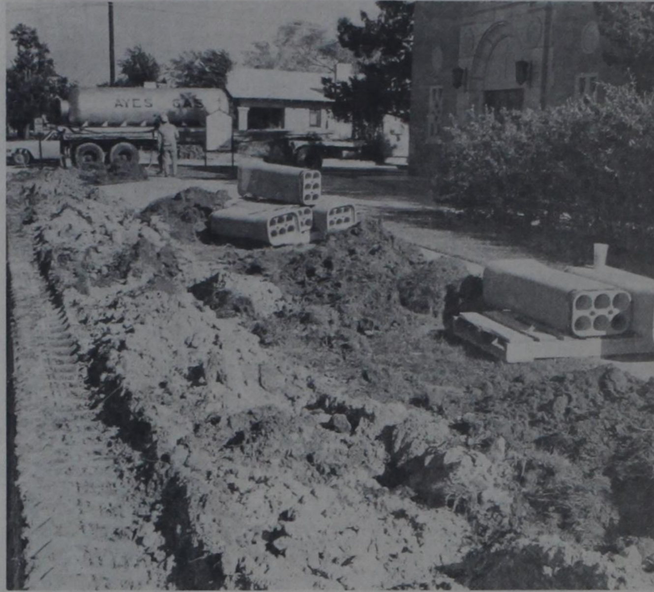
CONTRACTORS START WORK-Work has begun on Main street by contractors who are laying concrete conduits which will house the telephone cables going in and out of the Tech campus.
