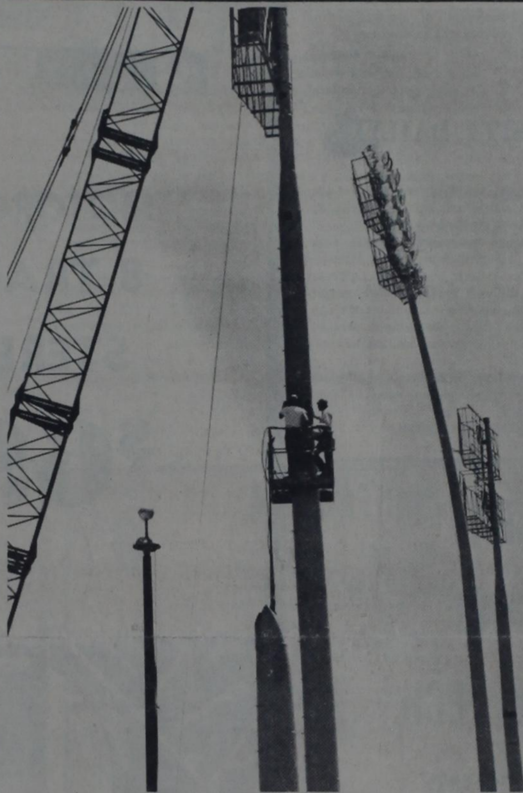
TWO FOR THREE—Workmen finish installing the second of two light poles at Jones Stadium to temporarily replace the three that were blown down in the May 11 tornado. The other new pole, finished Tuesday, is at the far right. Lights for the poles are expected to be installed and tested by June 24, three days before the Coaches' All-America Game. (Staff Photo by Bruce Ott)
