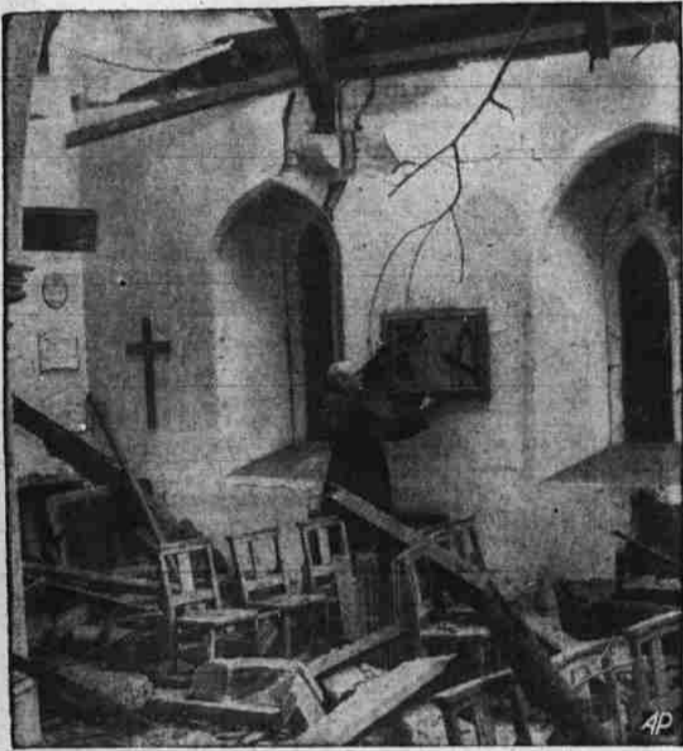
WAR RUIN —The Vicar removes one of the stations of the cross which, with the crucifix at left, remained intact when his church was practically demolished during a raid on the London area. Note that the force of the bomb has blown off the roof.
