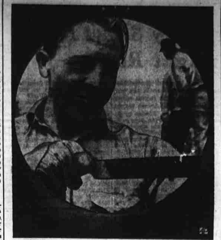
INSIDE STUFF—Intently a workman files the end of 12 1/2-inch pipe, before welding, on the $5,000,000 Portland, Mo., to Montreal oil pipe line being built. Overland pipe route will save tankers' 12 days' passage in the St. Lawrence.
