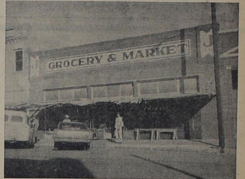
Morgan "Foggie" Bennett standing under the old awning at Jay's Grocery which he helped to tear down to make way for the "NEW LOOK". Morgan helped erect this awning about 28 years ago.
