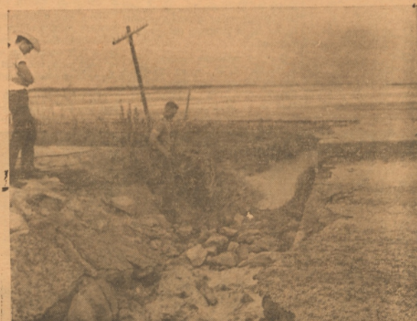
WASHED-OUT BRIDGE ON KOKOMO ROAD EAST OF CARBON WITH DAMAGED FARM LAND IN BACKGROUND
