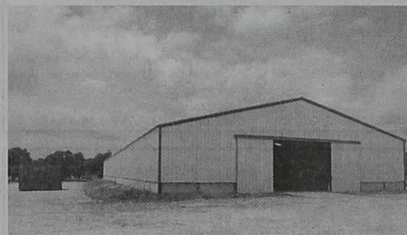
The new Pellet Mill Building for Gorman Milling is still under construction. Campbell Construction is working on the building.
