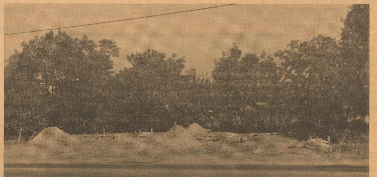
Foundation of the new home of Mr. and Mrs. D. O. Munn has been poured and construction will begin within a short time. Building materials and furnishings by Higginbotham's. A. L. Williamson and Dean Bennett are the builders
