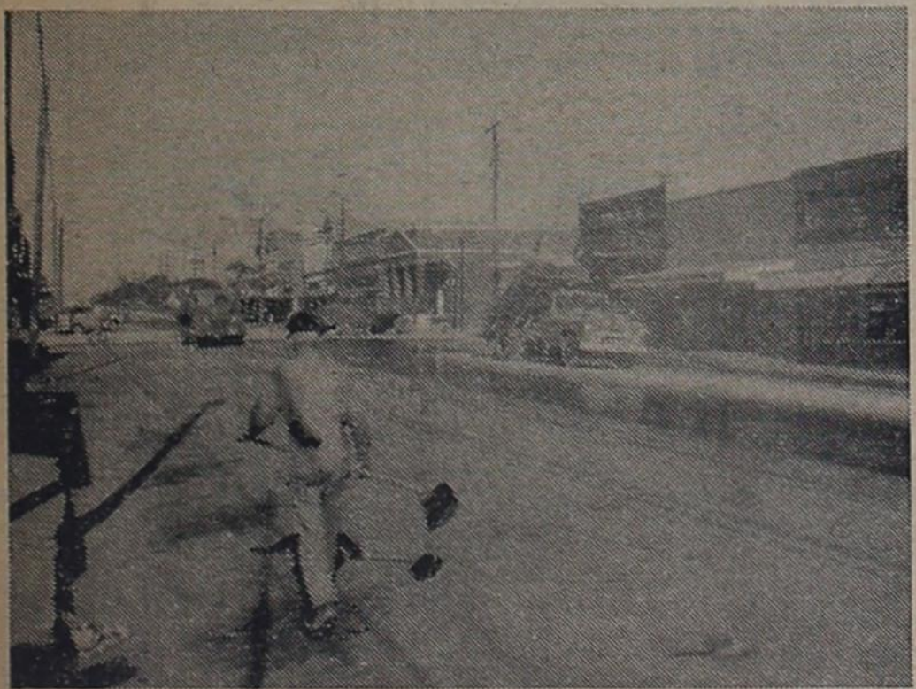
NEW TOPPING — This picture was taken Sunday as city employees finished the job of topping Kent Street and Roberts Street. Work is also being done on other streets. (Rex Yarbrough got caught in the picture).
