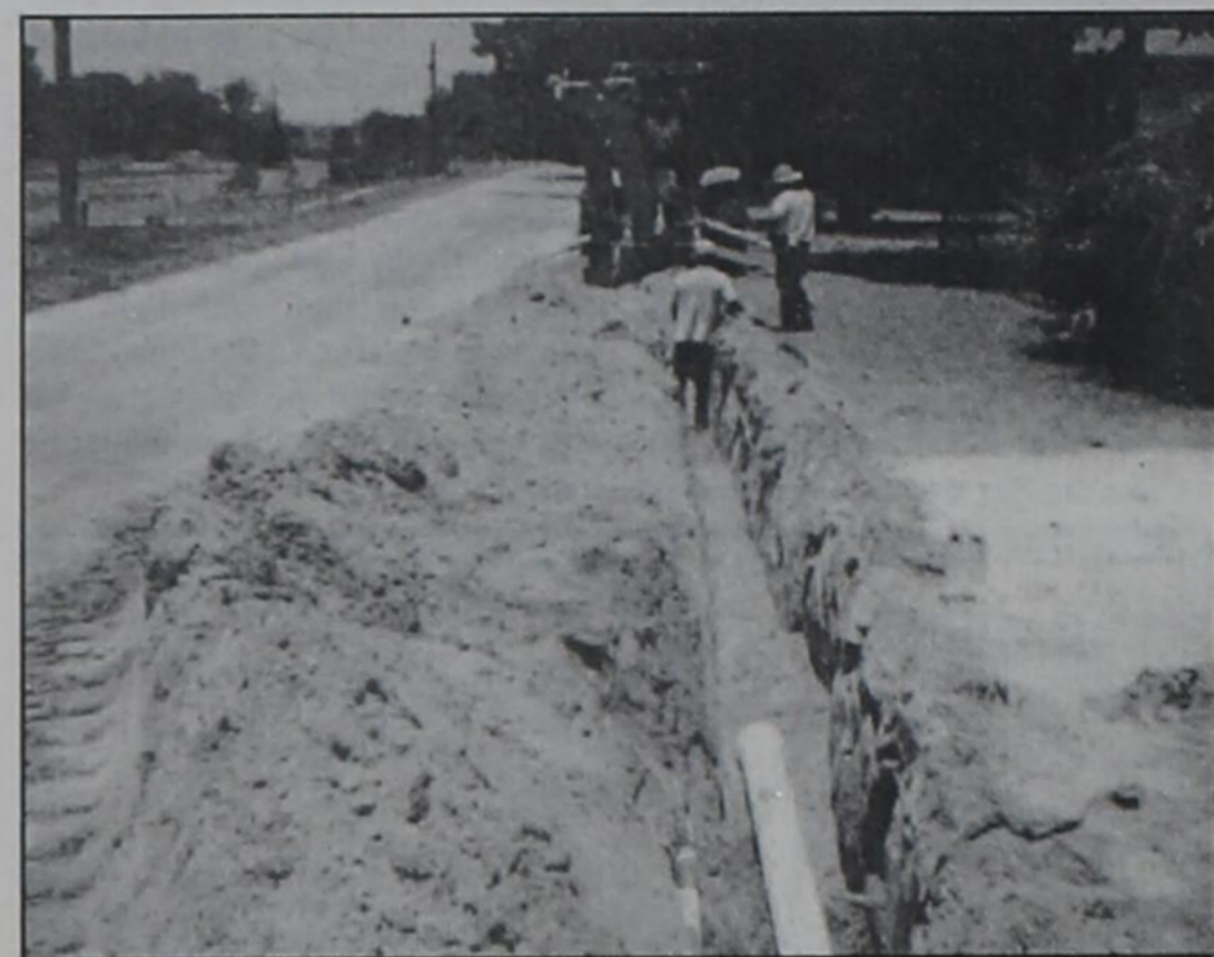
NEW WATER LINES — Works are shown digging the trench for the new water lines being installed in Gorman. The new lines will enlarge the water capacity and several new fire hydrants are being installed.
