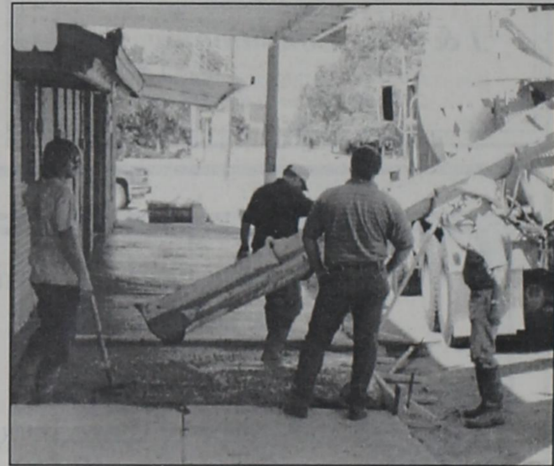
POURING NEW SIDEWALKS — Bimbo Roberts Concrete crew is shown pouring the last section of the new sidewalk in front of the City Hall. All the sidewalks on the East side of main street will be replaced later. This helps the look of our downtown and is safer for the citizens and visitors to Gorman.
