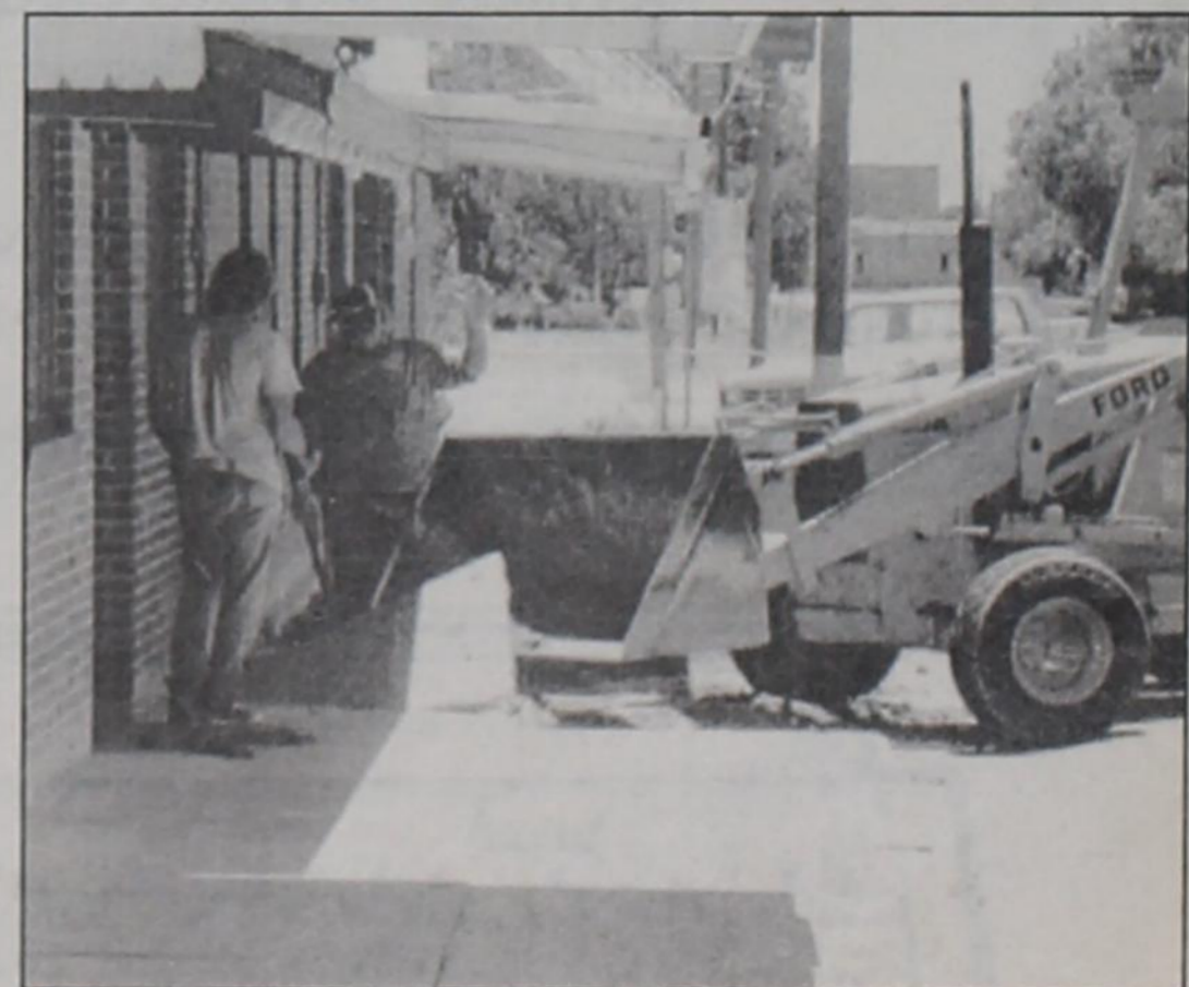
BUSTING UP SIDEWALKS — Shown above is the city crew breaking up the sidewalk in front of the City Hall and Village Crafts. The old concrete sidewalk was removed to make way for a new and better sidewalk.
