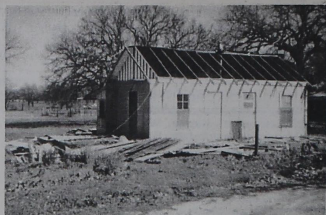
ANOTHER LANDMARK GOING DOWN — The old Cass Clark home on the curve near the swimming pool is hown being torn down this week. We didn't know any other details of this project at this time. This was one of the older homes in Gorman.
