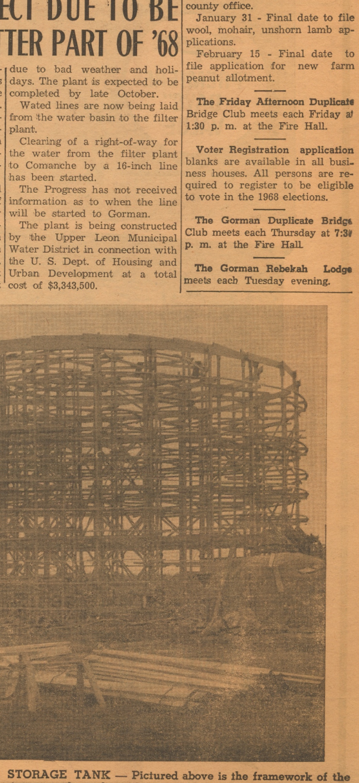
MILLION DOLLAR WATER STORAGE TANK — Pictured above is the framework of the new one million gallon water storage tank at the new water treatment plant now under construction at Proctor Dam.
