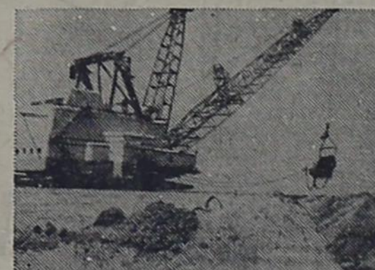
First, the overburden, which is from 40 to 130 feet deep, is removed by this giant dragline.
