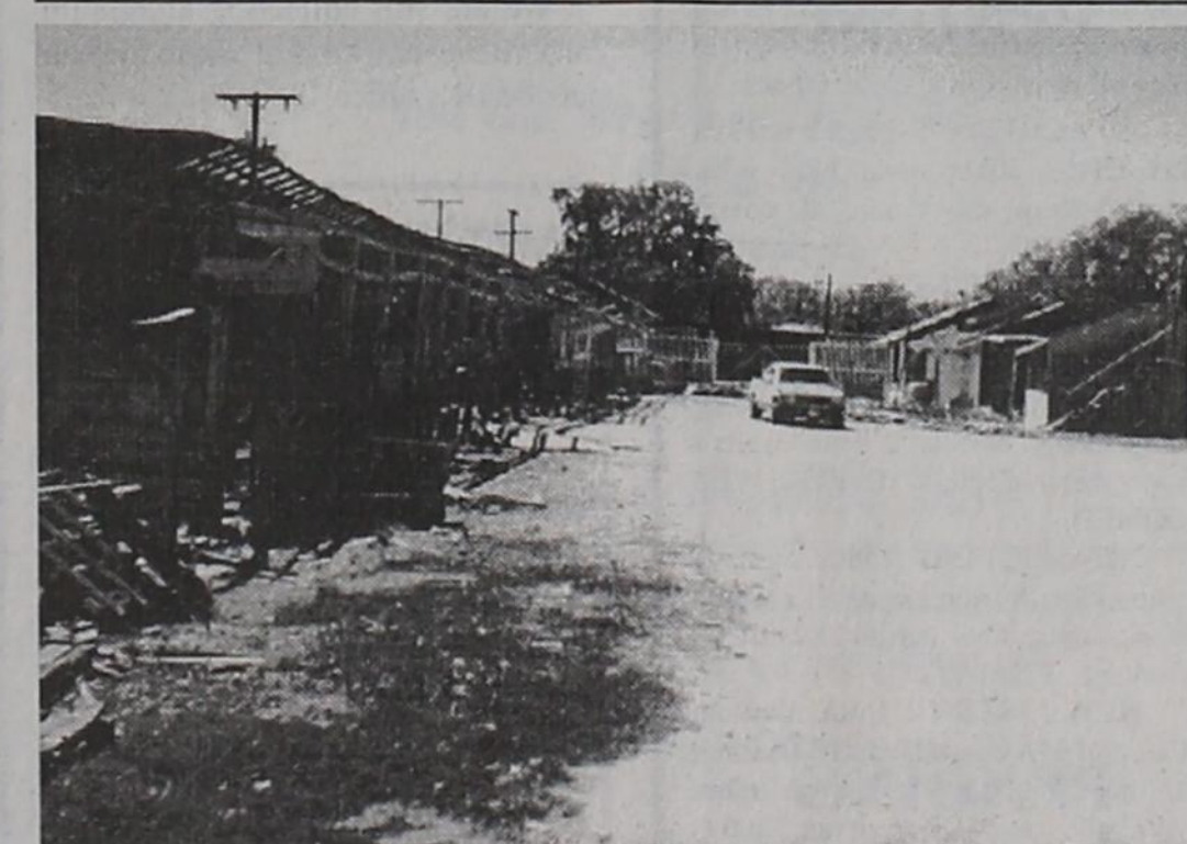
DEMOLITION OF LUMBER YARD — The above picture shows the demolition of the old Higginbotham's Lumber Yard buildings located close to downtown in Gorman. The buildings have been in Gorman for many years. The Lumber yard closed about a year ago when it merged with the De Leon Higginbotham Lumber Yard.
