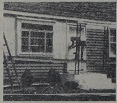
8. INSULATION BOARD — The lightweight insulating panels are nailed over the old exterior, providing a solid backing for the new siding.
