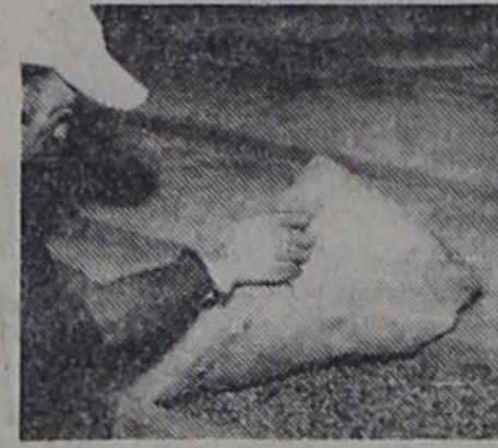
1. INSULATE — A minimum of 6" thick R-19 fiber glass insulation in the attic can reduce fuel consumption up to 30%.
