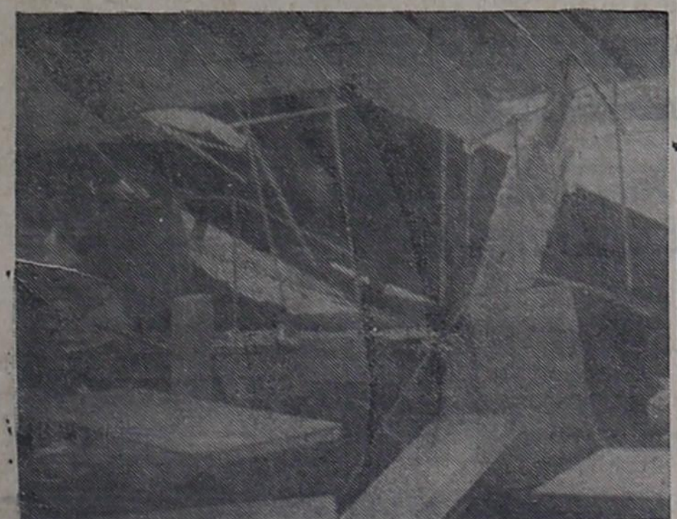
WEATHER DAMAGE — This photo shows part of the very heavy damage to the Ray Williams building in the downtown area of Gorman during last weeks wind, hail and water deluge. The back section of the roof collapsed.
