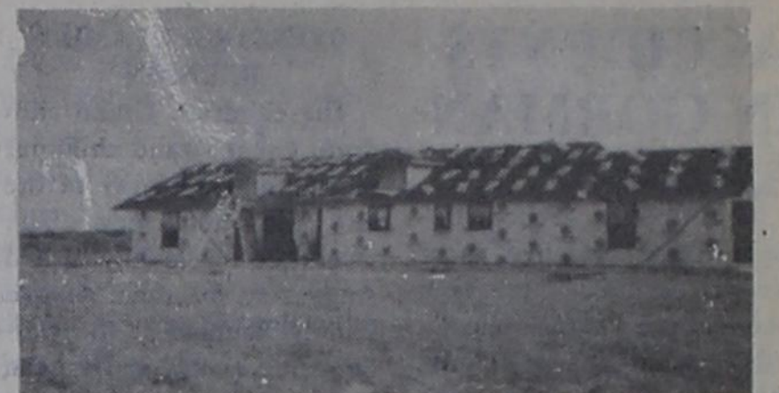
ANOTHER NEW HOME-- Shown above is the new home of James and Ann Jay under construction on the Desdemons highway. Completion is expected soon.
