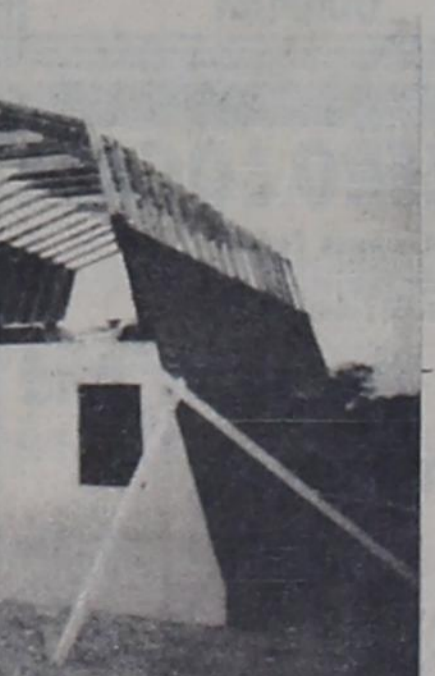
NEW HOME UNDER CONSTRUCTION — The Home of C. W. Swanner is being built in the south east section of town. This is a self constructed project by the family.
