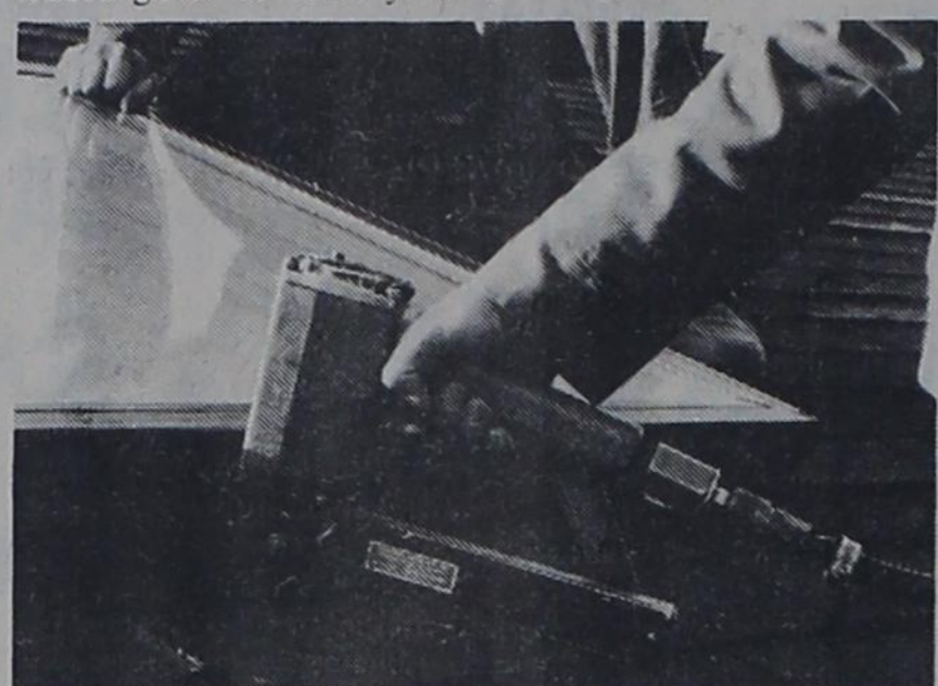
The key to installing a skylight is to flush it properly with the roof so that it doesn't leak later, says this Duo-Fast expert. A pneumatic roofing stapler can speed work also.
