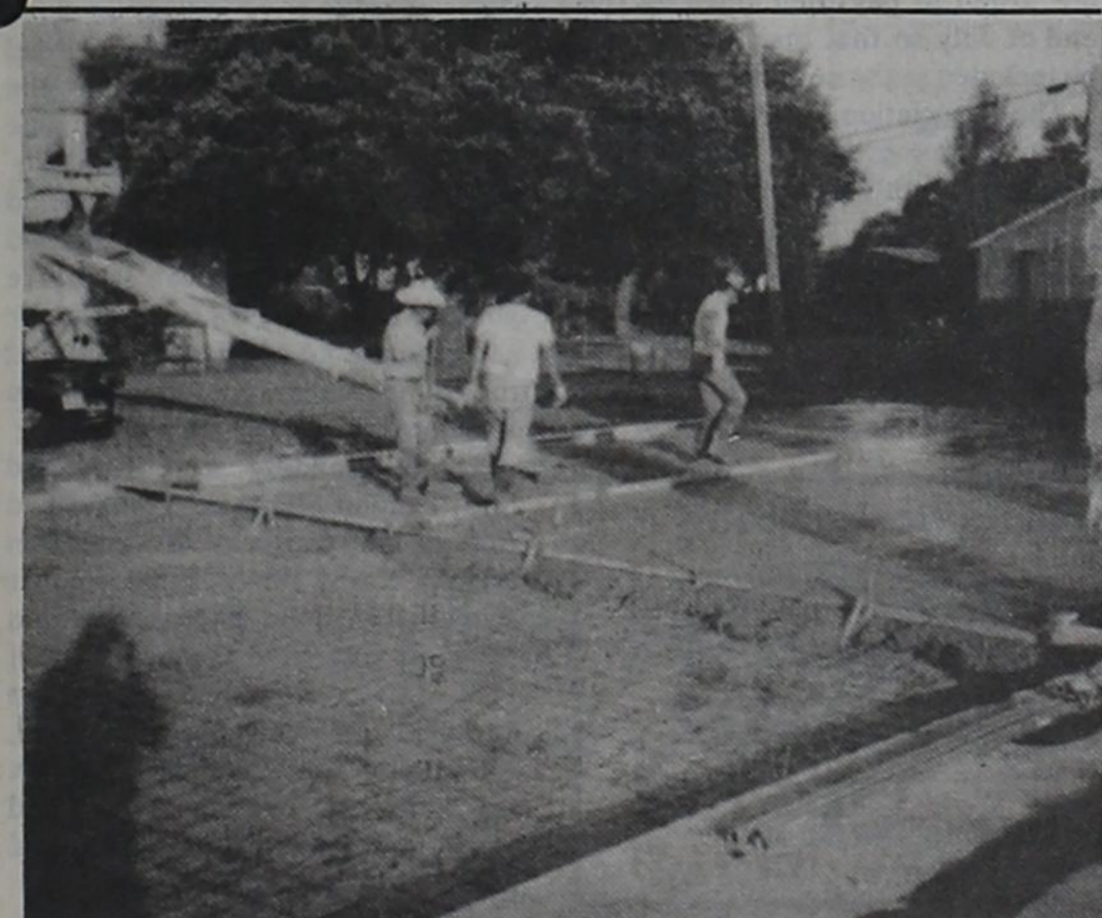
ONGOING WORK - The concrete work on the new add-on at the Gorman Fire Department Building was done late last week. The concrete work is being done by the Tommy Roberts crew.
