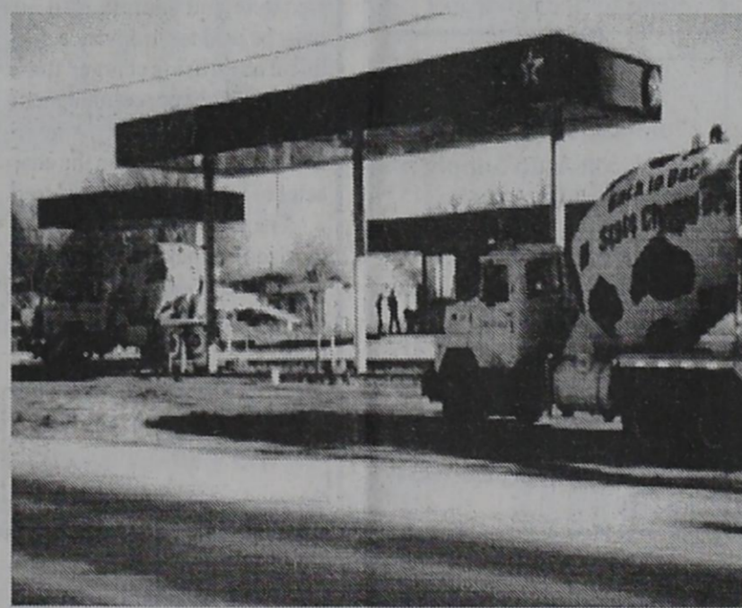
CONCRETE WORK CONTINUES -- The concrete work continues on the new Texaco Convenience Store being built in Gorman across from SWPGA.
