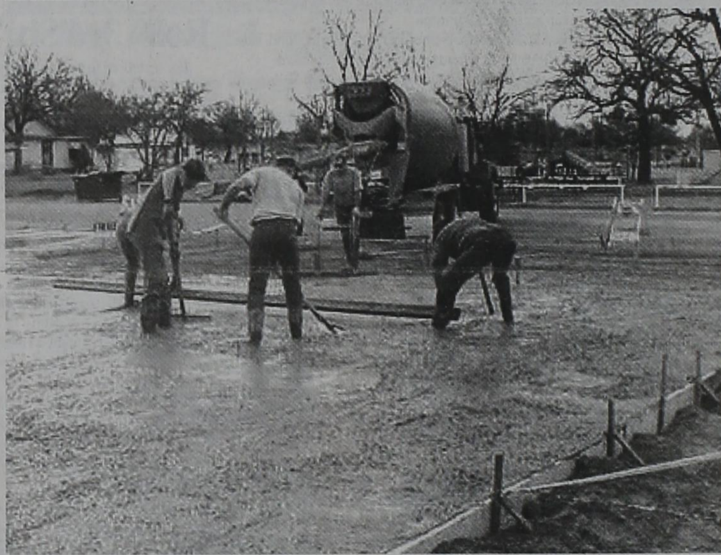
CONCRETE BEING LAID - Above are several local concrete workers laying the floor for the new basketball half courts being constructed in downtown Gorman next to the Senior Citizens Building.
