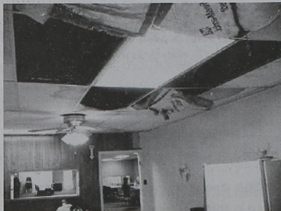
Ceiling in Senior Citizens Center in Need Of Repairs. The roof was repaired last week.
