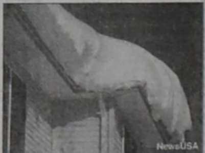
Snow buildup can result in water damage, which leaves your home open to pests.
