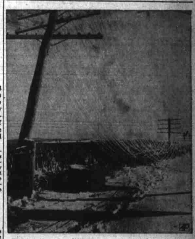
Wires Sag Under Ice Load—Telephone and telegraph wires sagged under the weight of snow and ice which left up to six inches of snow in eastern Nebraska and western Iowa. The Northwestern Bell company sent a crew of 500 into the storm area.
