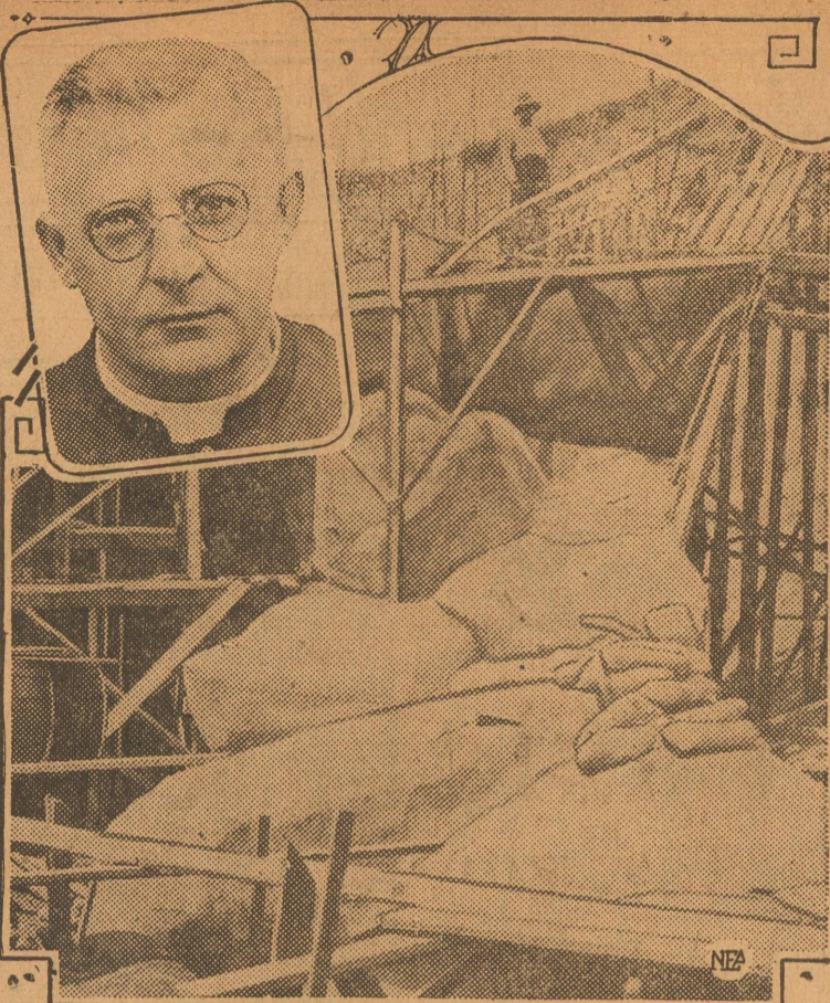
An exact duplicate of the famous Lourdes Grotto of France, where many miraculous cures are reported annually, is being built by the congregation of St. Joseph's church at St. Joseph, O. This picture shows the grotto under construction; inset is Rev. Edward J. Spitzig, pastor of the church and supervisor of the work.
