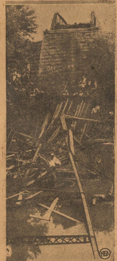
A 174-foot bridge span collapsed and dropped forty feet into the Verdigris river, near Coffeyville, Kas., when they tried to move a thirty-ton oil well drill across it. Two men were drowned and three others seriously injured.
