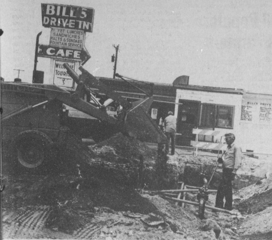
PUTTING IN THE PIPES AND TANKS--At the location of the new Town and Country Convenience Store, workmen have been installing gas tanks and gas pipes. The workmen are from Lubbock and said they will be installing pumps in the near future.
