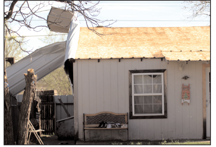
Hector and Lisa Guevara had flooding and the roof ripped off their house.
