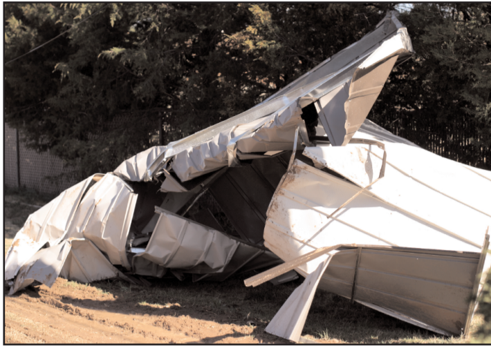
This garage was wrapped around a set of power lines, but the electric company came out and cut it off.
