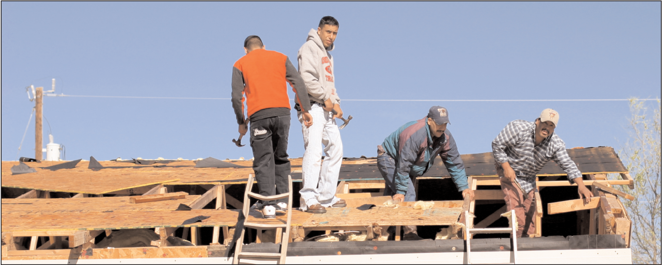
Bovina's Cornelio Ortiz starts the work of replacing a roof that was destroyed by the storm.
