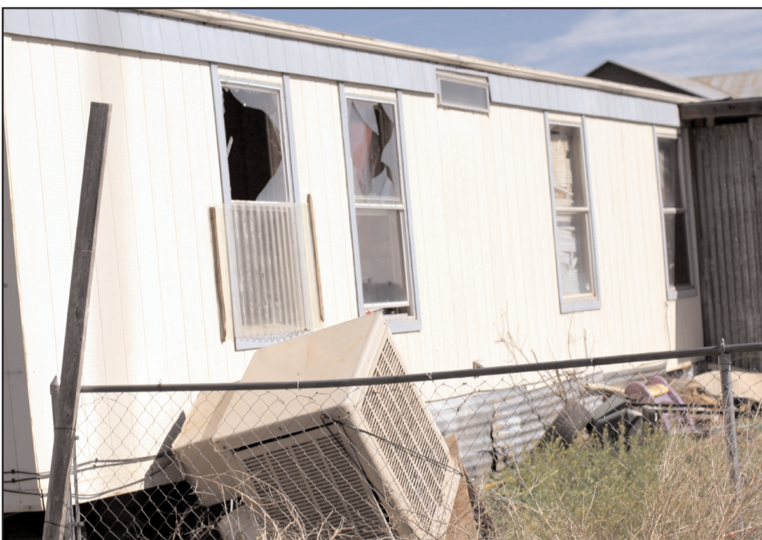
Bovina's Valerie Elias had some windows broken and roof damage. Her 6 year old son Gabriel humorously pointed out the damage done by the "toma-to".
