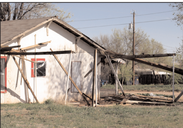
Eddie Garcia Jr. had his car repaired last week and parked it under his carport for the storm. The carport was destroyed, but the car was undamaged.
