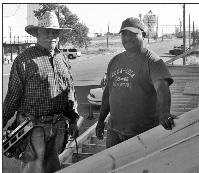
Lazaro Munoz and his son Luis Carlos, atop the construction project at Bovina City Hall, anticipate its completion within two weeks.
