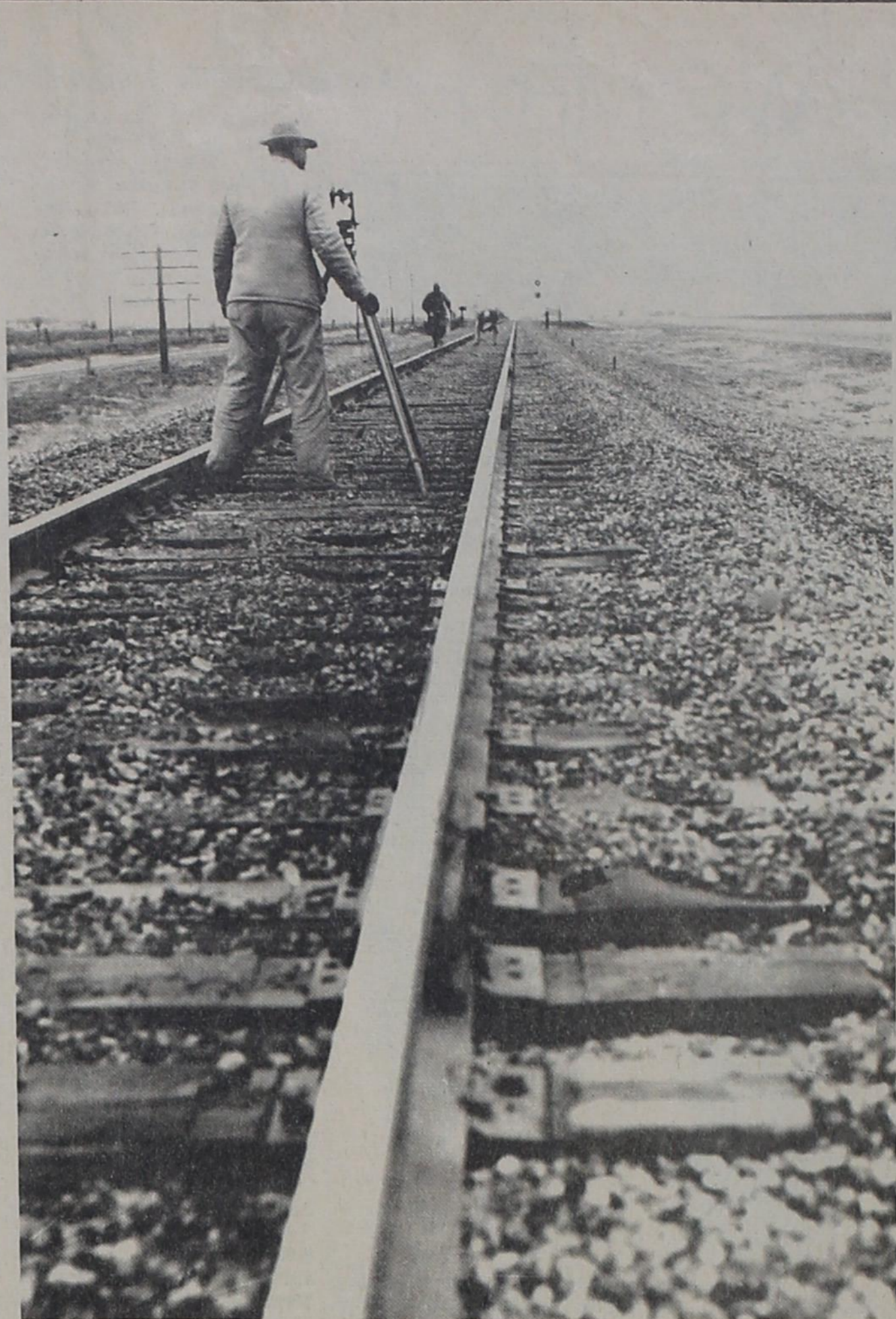
I'VE BEEN WORKIN' ON THE RAILROAD---Engineers hurry to complete their "shots" with an optical levelling instrument on the new ballast and track on the Amarillo line just a short ways out of town. Major maintenance work has been going on recently. Less than ten seconds after this picture was made the men scurried off the track to make way for a thundering train.
