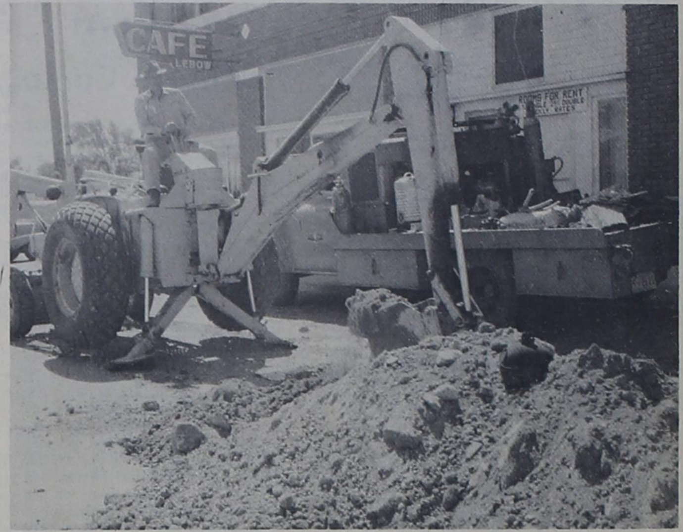
Employees of Southern Union Gas Co. were busy in the Twin Cities this week repairing gas lines and seeking out minute leaks which might cause trouble. One might think with the continued heat wave "who needs gas", however in a few short weeks residents of the town will be making pleas for the company employees to hurry-hurry and get the gas on before we freeze.
