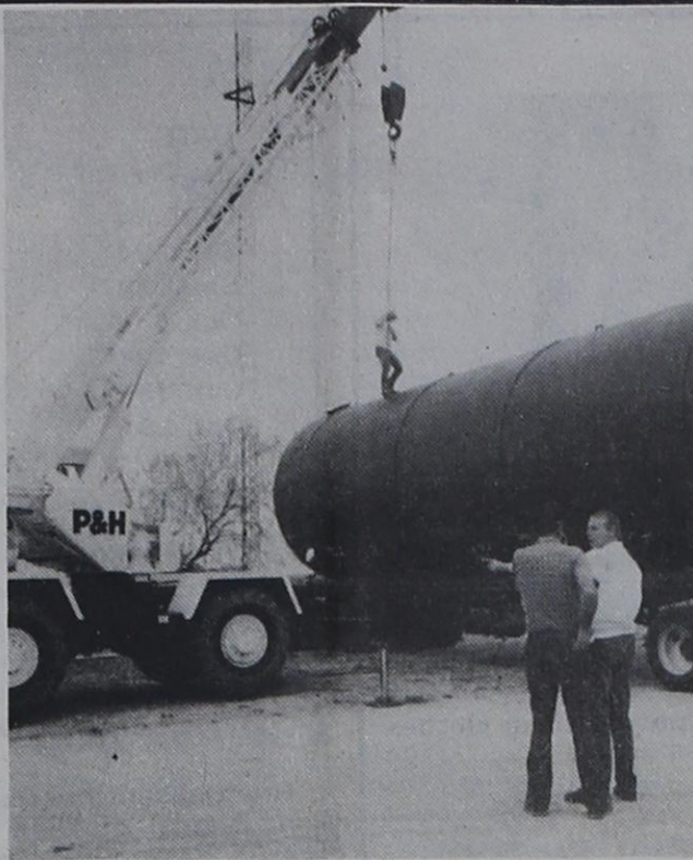
Bill Servatius climbed atop the tank to fasten the guide wires while Richard Kelley and Paul D. Barnes discussed operations from the ground.
