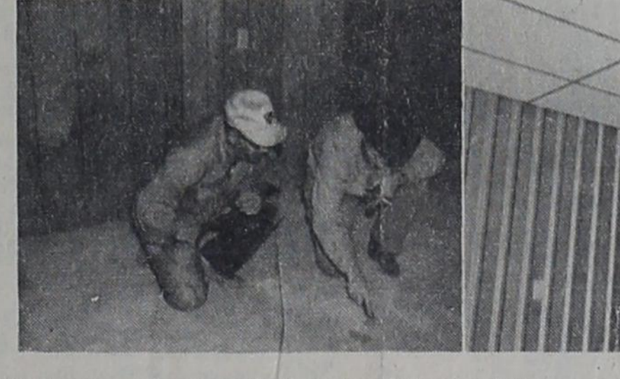
Workmen are busy on the interior of the new dining room of Clara's AA Bowl Cafe, located at the AA Bowl. Pictures show the paneling which extends on the lower half of the wall, and the ceiling design.
